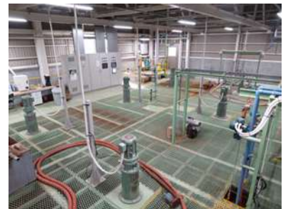
Upgraded pit wastewater treatment facility (Osarizawa Mine)
