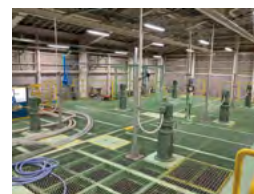
Mine drainage treatment facility (upgraded) (Komagi Mine)
