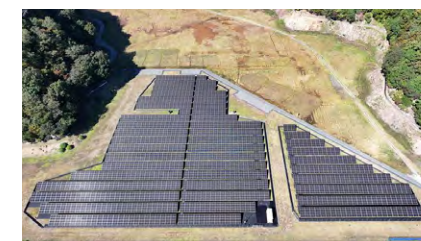
Torinooku Solar Power Plant
